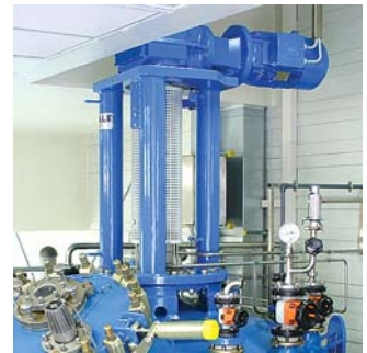
Reactor BE 8 m 3 with agitator drive TRD 500 / 7,5 / 10 kW – SX in operation at Serumwerk Bernburg GmbH
